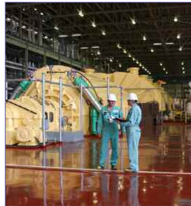
The Bruce A turbine hall.
